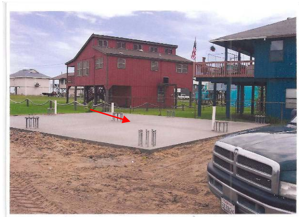
Figure 8.3-4. Construction photograph shows 24-inch deep bolts extending into the cement foundation (red arrow). The slab extends over the outside concrete foundation. Photo courtesy of Ron Bell.
