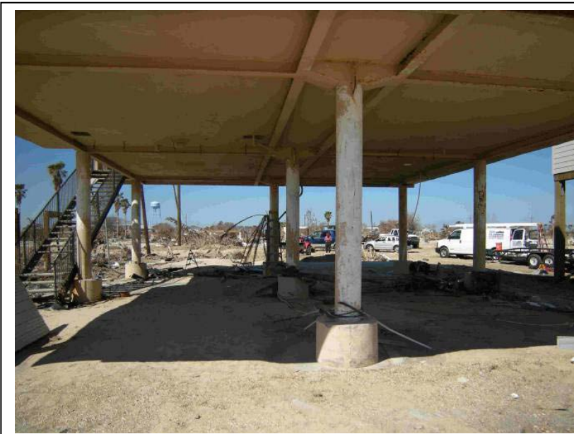
Figure 8.3-11. (101808d- 3688) View looking north under the house. Foundation of the Crystal Beach SCIP house did not sustain damage from Hurricane Ike.
