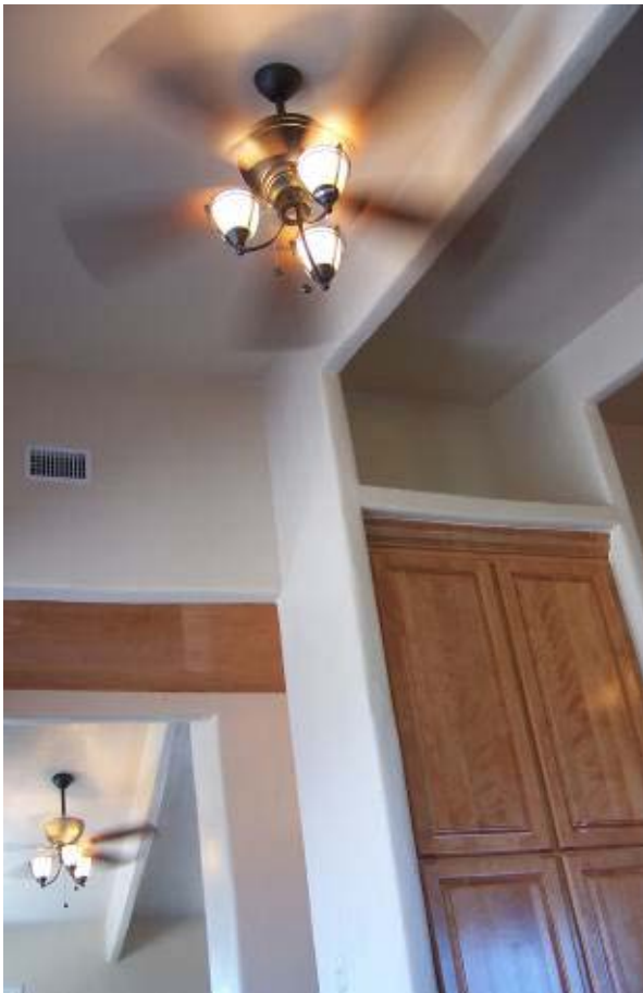
Figure 8.3-6. The roof SCIP beams are shown above the fans, following the roof slope. The 18-inch deep beams are tied into the 30-inch deep columns that are vertical members in this photograph. The Crystal Beach House used No. 14 gauge wire frame.
