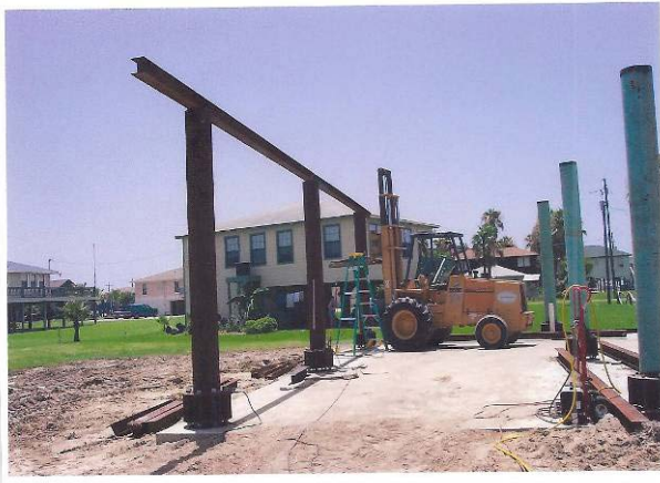
Figure 8.3-5. Construction photograph shows columns bolted in place. The nuts under the flange are used to level the 6-foot by 6-foot H beam. The rebar that will extend into the first floor vertical walls will be welded to the first floor (elevated) beam shown in the photograph. Photo courtesy of Ron Bell.
