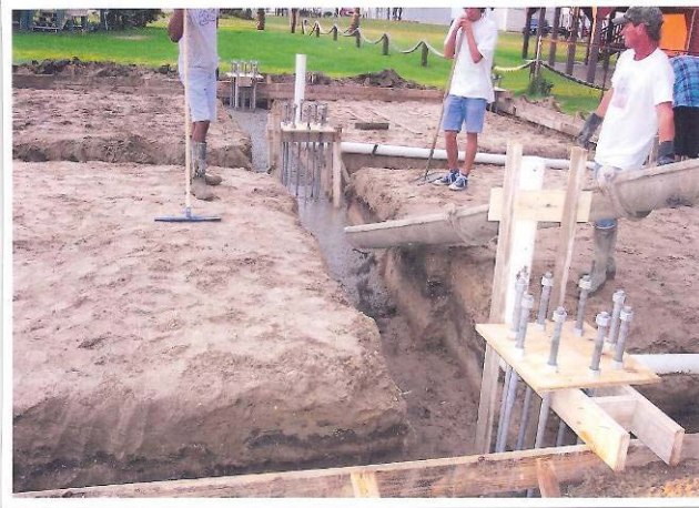
Figure 8.3-3. Construction photograph shows foundation with nine sets of bolts for the columns. There is a perimeter-grade beam and a center-grade beam. The men on the right are standing on sand at the height of the 6-inch slab. Photo courtesy of Ron Bell
